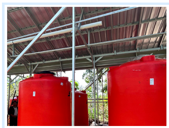
Rainwater storage for the Smart Mist Irrigation system in Temon Sub-village, Giripurwo Village, Purwosari District, Gunungkidul Regency. Photo: Nanda/YEU
